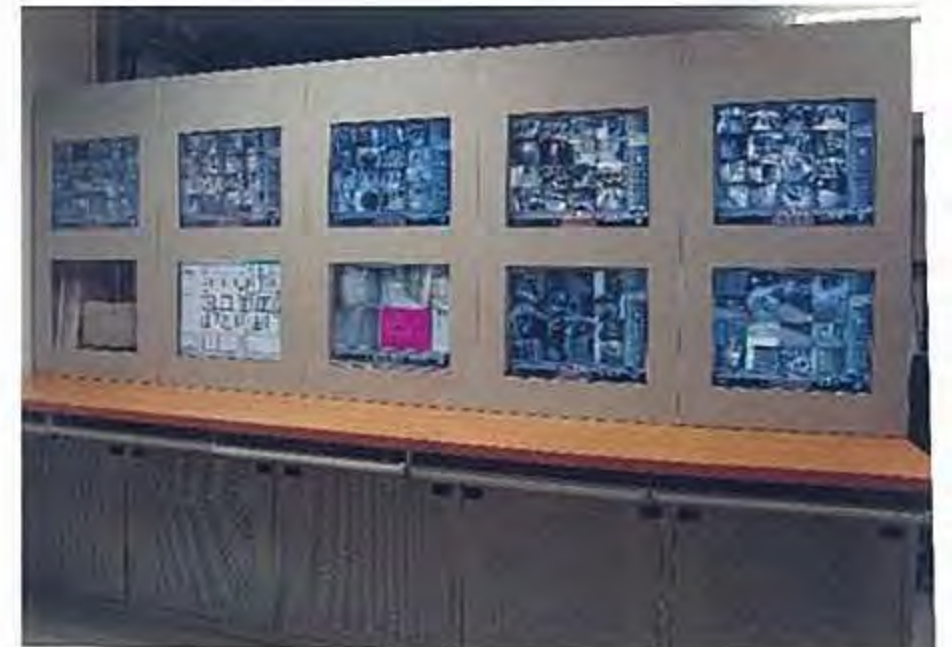
機場監控牆 Airport Monitoring Console
